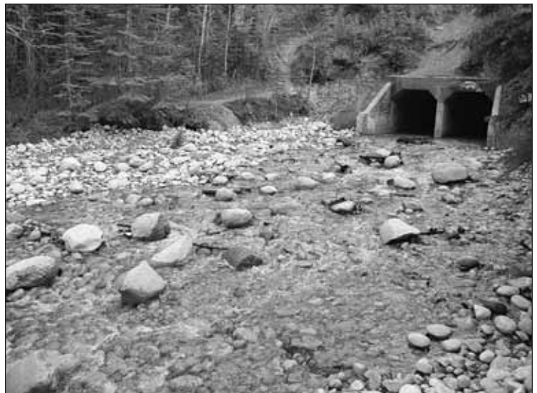
Canadian National Railways culvert on Hardisty Creek prior to remediation.
