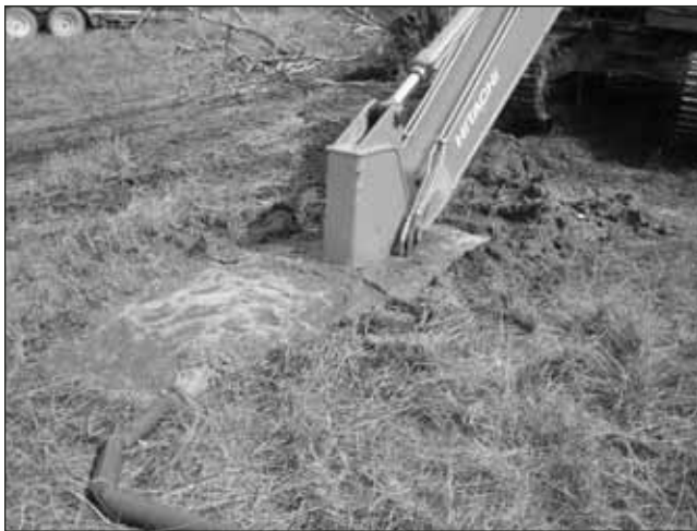
Keeping the hole full of water during the backhoe digging operation will prevent the sides from caving in.
